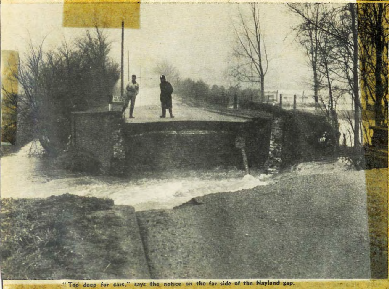
And Popps Bridge is no more. A twenty-five yard gap divides Suffolk from Essex and will do until the Bailey bridge is complete.
